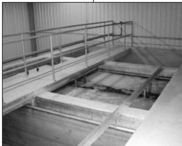
DISSOLVED AIR FLOTATION TANKS
