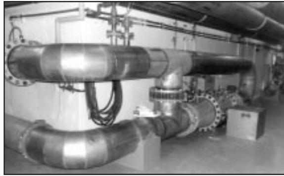
In Line Installation
