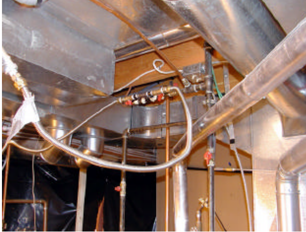
Unsupported flexible gas lines used to fuel CO 2 generators. (Photo 12)
