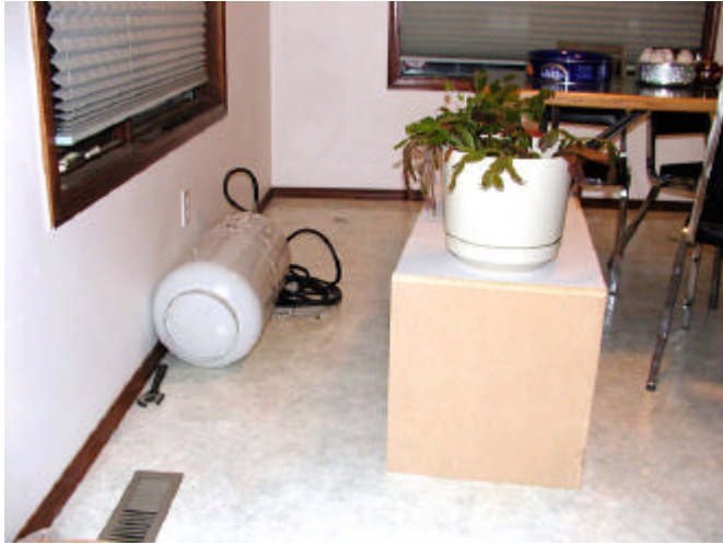
A 30 lb propane cylinder lying on its side, found concealed underneath a bench seat in the kitchen. The gas line ran through the floor to a CO 2 generator below. (Photo 15)
