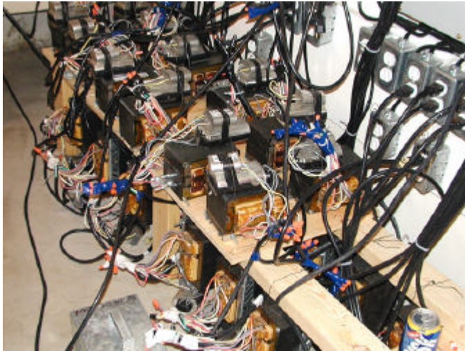
Maze of 220VAC supply lines to the transformers used to power the high intensity grow lamps. ( Photo 7 )
