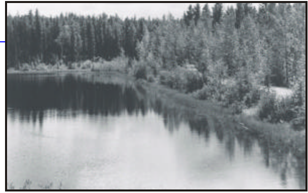
Photo No. 5 (DSB 9200-40) Pedley Water Tank, 1976 Excessive vegetation on upstream slope.
