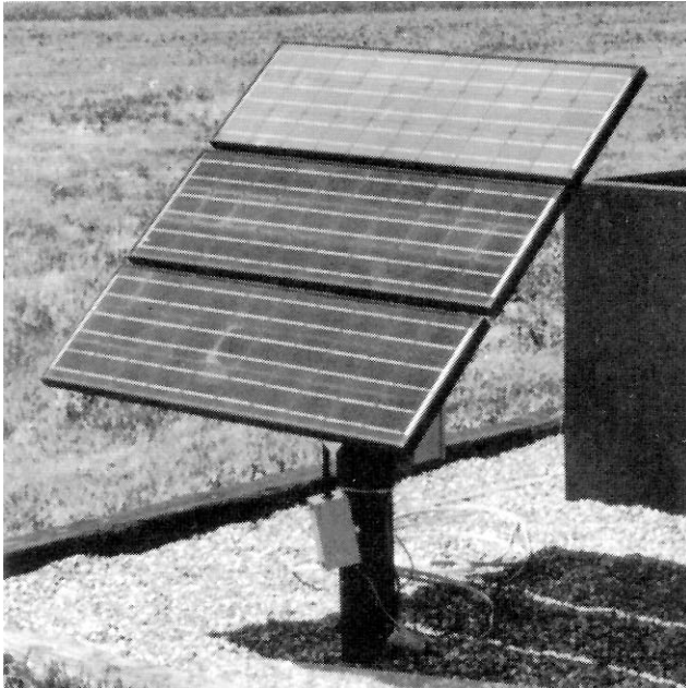
FIGURE 1. Cap 3 Solar Panel
