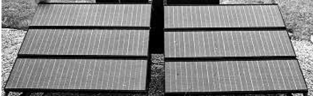
Figure 1. Kelln 6 Module Water System (Parallel/Series).
