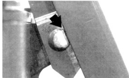
FIGURE 6. Interference between Pump Handle and Rivet.
