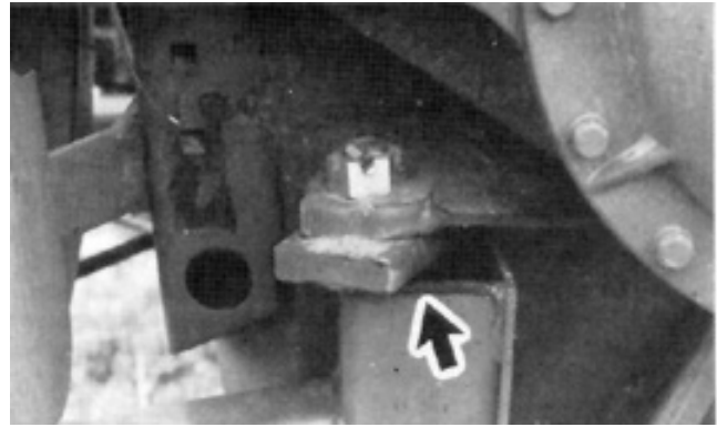
FIGURE 8. Broken Hitch Weld.
