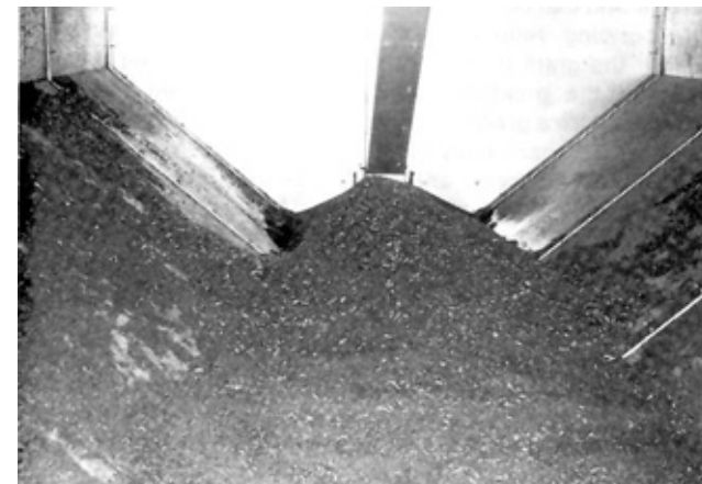
FIGURE 10. Accumulation of Fines in the Cool Air Plenum.
