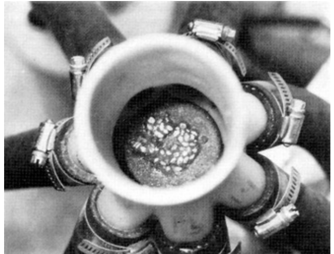
FIGURE 19. Moist Soil Build-up: (Upper: Primary Header, Lower: Secondary Header).
