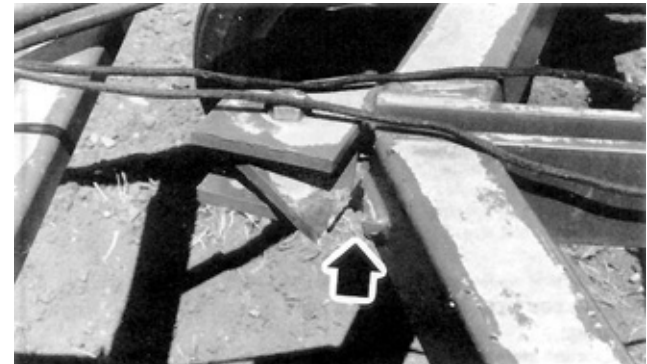
FIGURE 26. Front Pivot Joint Failure.
