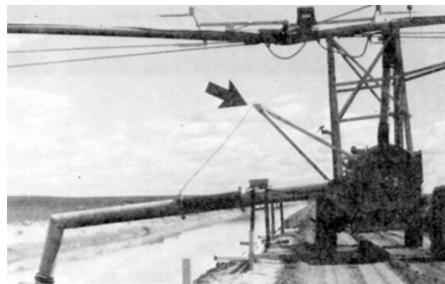
FIGURE 17. Winch for Rainger Intake Float Level Adjustment.
