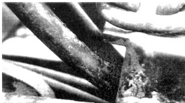
Figure 13. Damaged Depth and Wing Hydraulic Lines.
