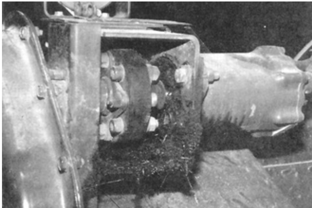
FIGURE 5. Leaking Oil Seal on Hydraulic Motor.
