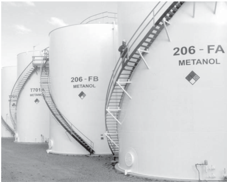
Methanex methanol storage tanks
