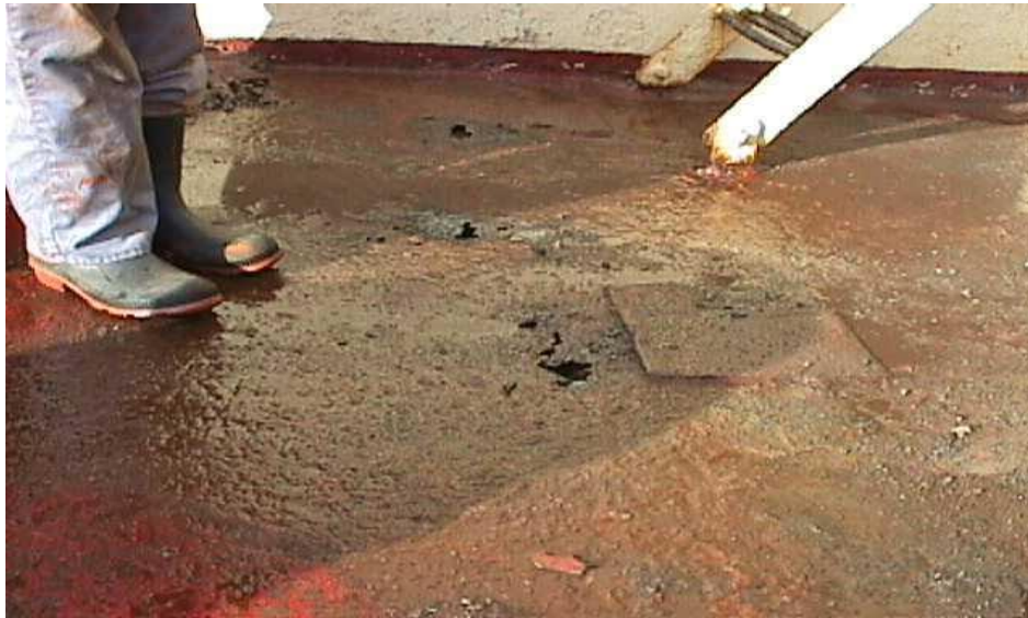
Deck plating corroded which could lead to serious consequences
