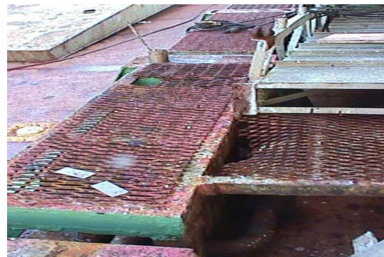
Deck grating corroded and holed
