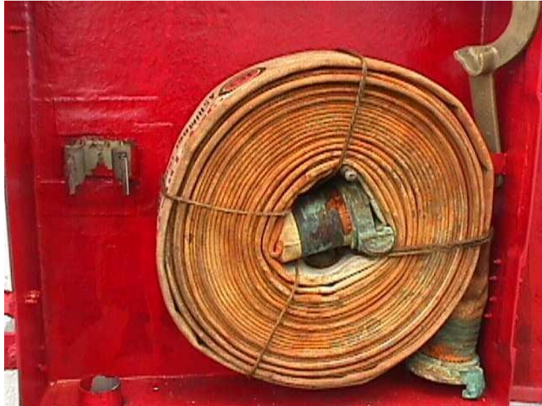
Tied up and corroded nozzles on firehoses
