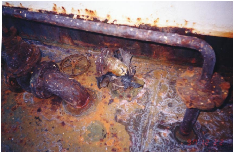
Poor maintenance often leads to the detention of foreign vessels
