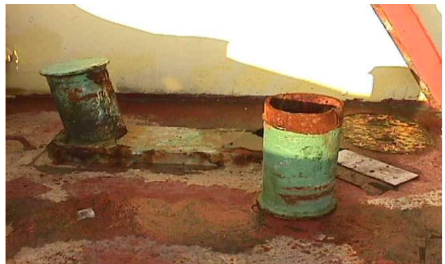
Corroded Mooring arrangement
