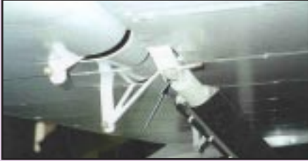
Upper end of a typical aft strut attaching the wing on a similar aircraft type.
