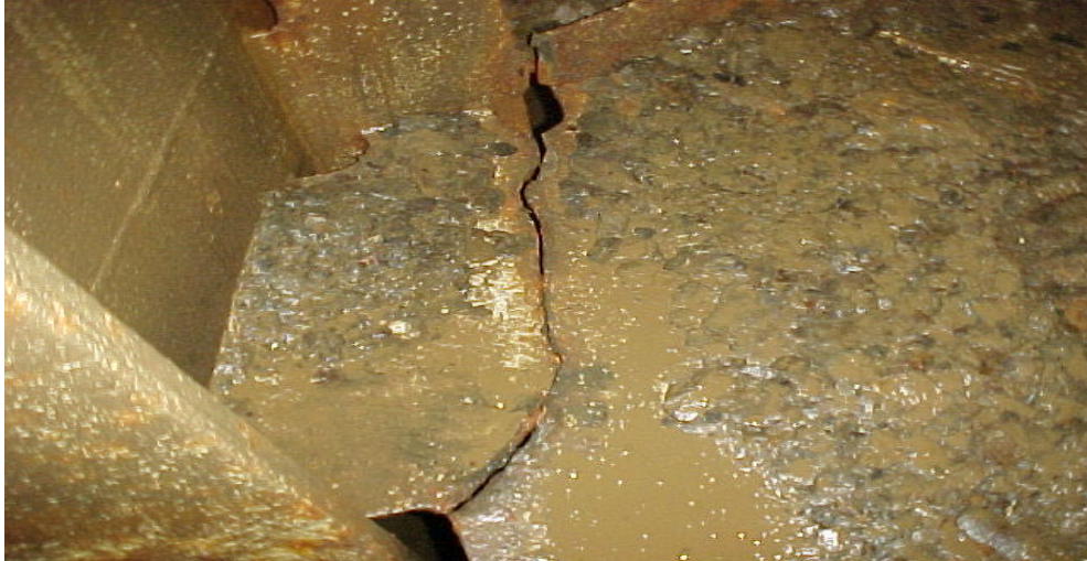
Severe corrosion found in way of the collision bulkhead inside the fore peak tank of a bulk carrier.
