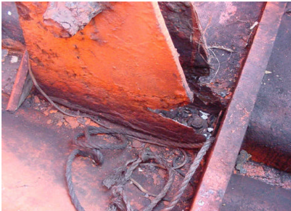
Lifeboat support bracket found heavily corroded during a port State control inspection.
