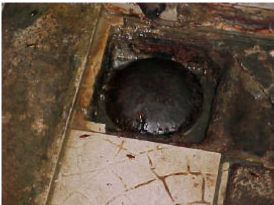
Galley drain filled with grease and infested with insects
