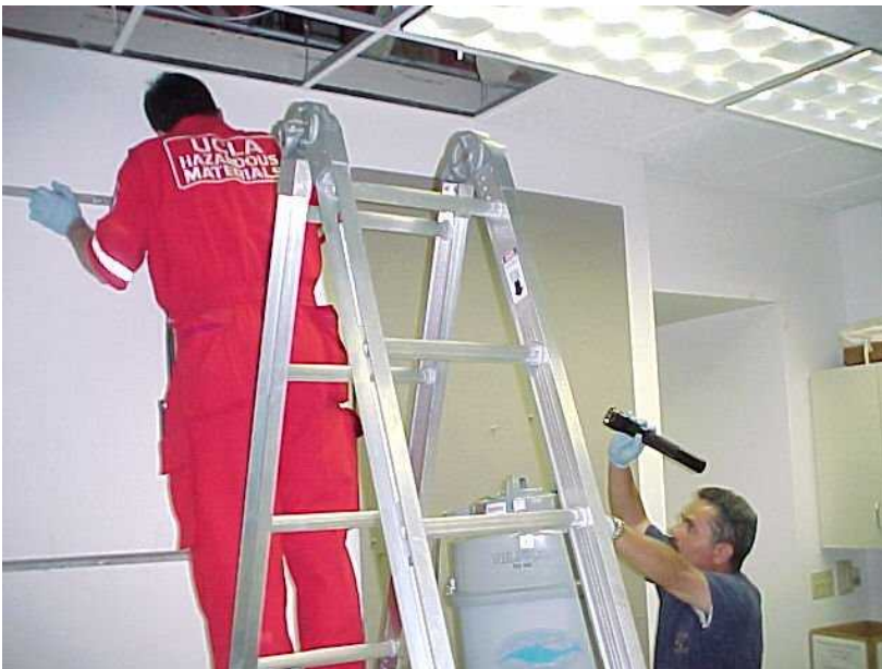
Figure 20 Investigating the extent of damage to ceiling tiles from a mercury spill. (Photograph courtesy of UCLA, Office of Environment, Health & Safety)
