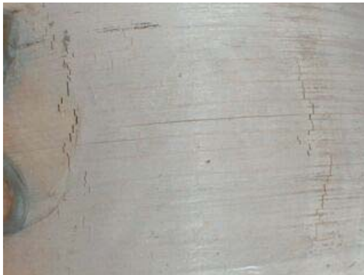
Figure 2: Damage to the Composite Wrapping
