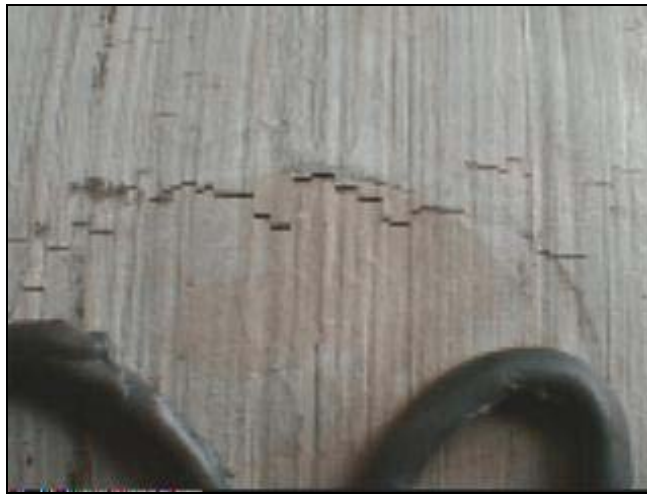
Figure 1: Damage to the Composite Wrapping
