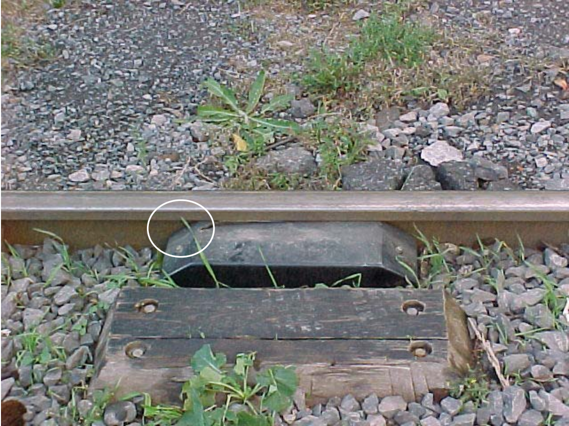
Figure 20 Speed sensor with damaged housing
