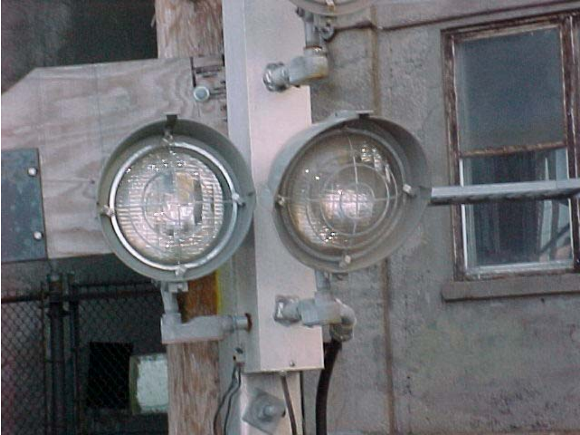
Figure 16 Spotlights (in position)
