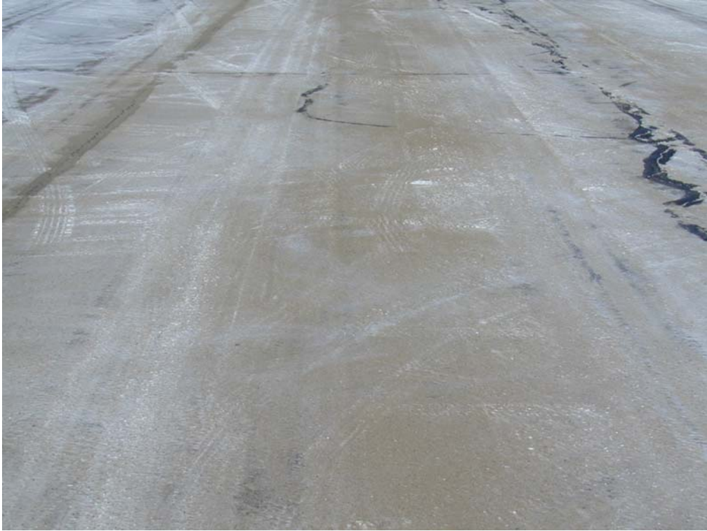
Figure 3.15: Sanded Partly Consolidated Snow on Pavement
