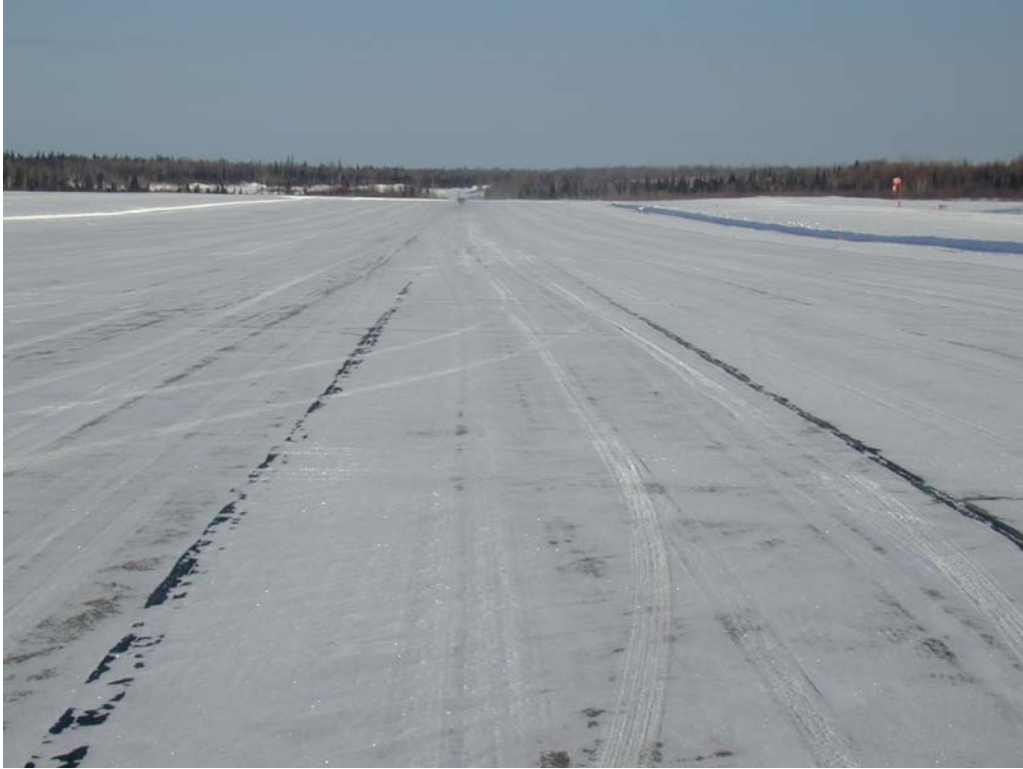
Figure 3.11: Loose Snow on Pavement
