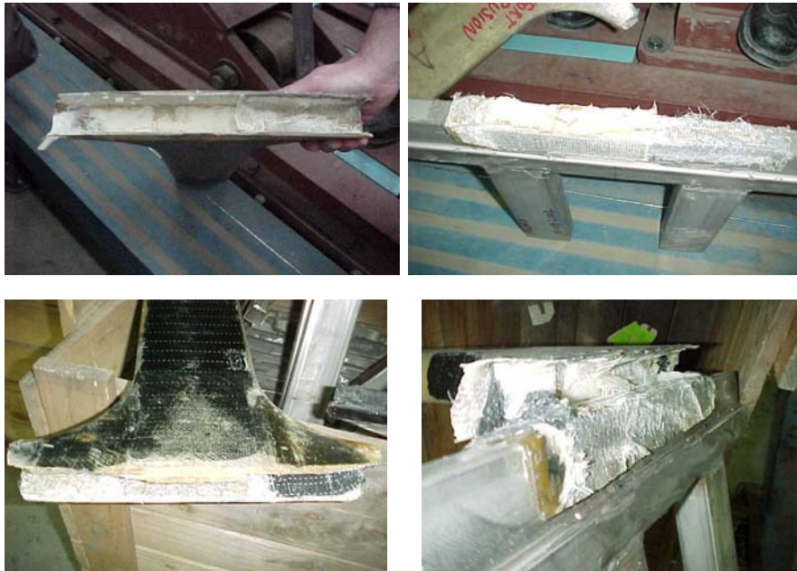
Figure 6.10: Examples of Post Failure
