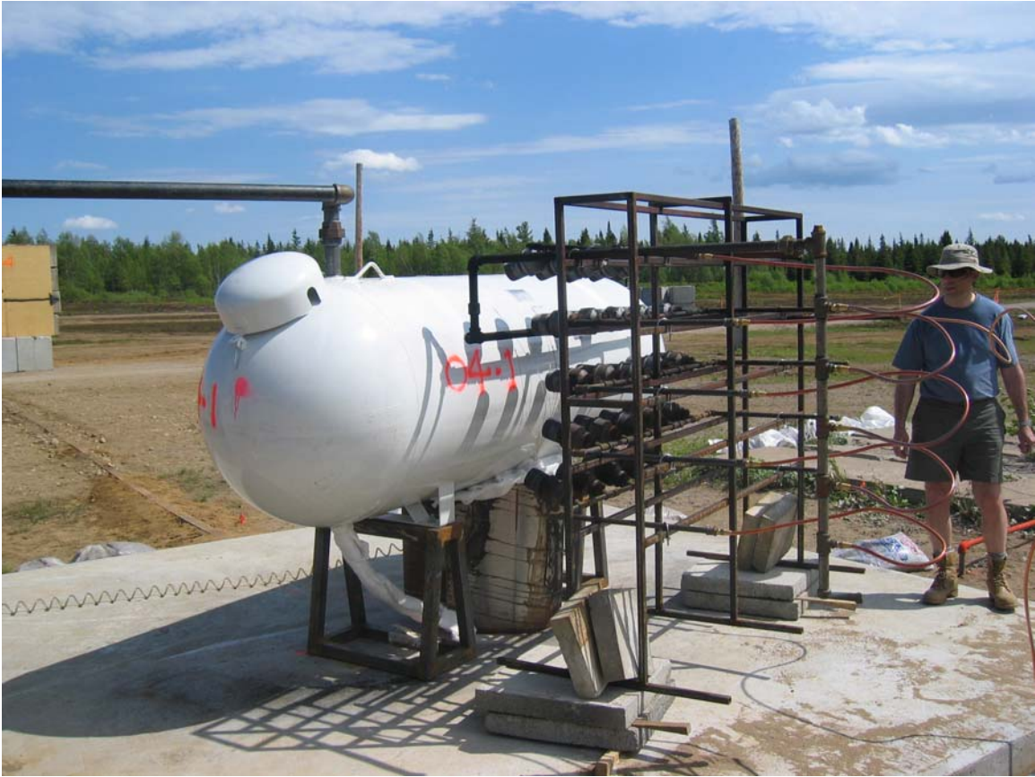
Figure 3.7: Tank 04-01 with burners in place
