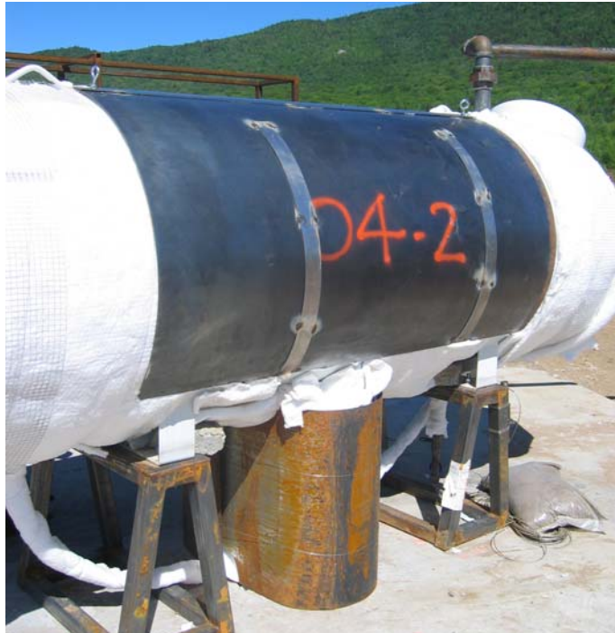
Figure 3: Test Tank Showing Jacketed Area (defect under jacket on other side of tank) [4]
