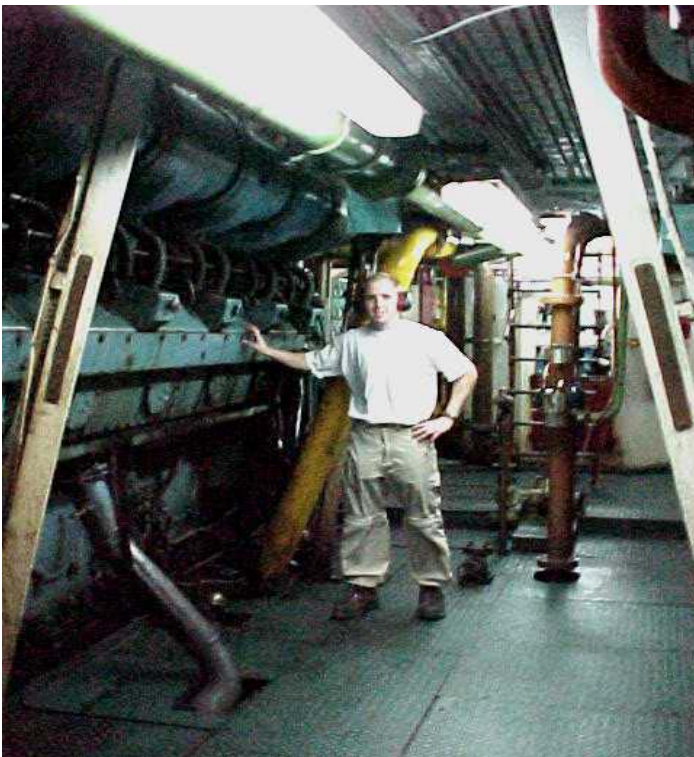
M.V. Cabot Engine Room (lower level)
