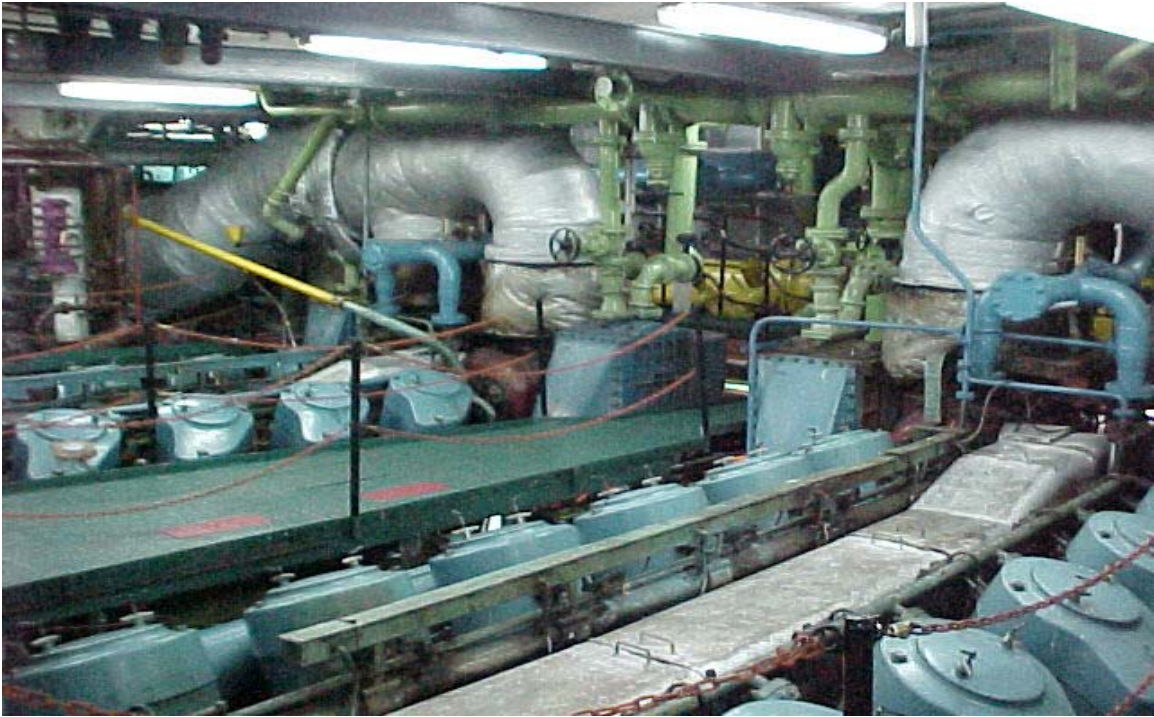
M.V. Cabot Engine Room (upper level, forward)
