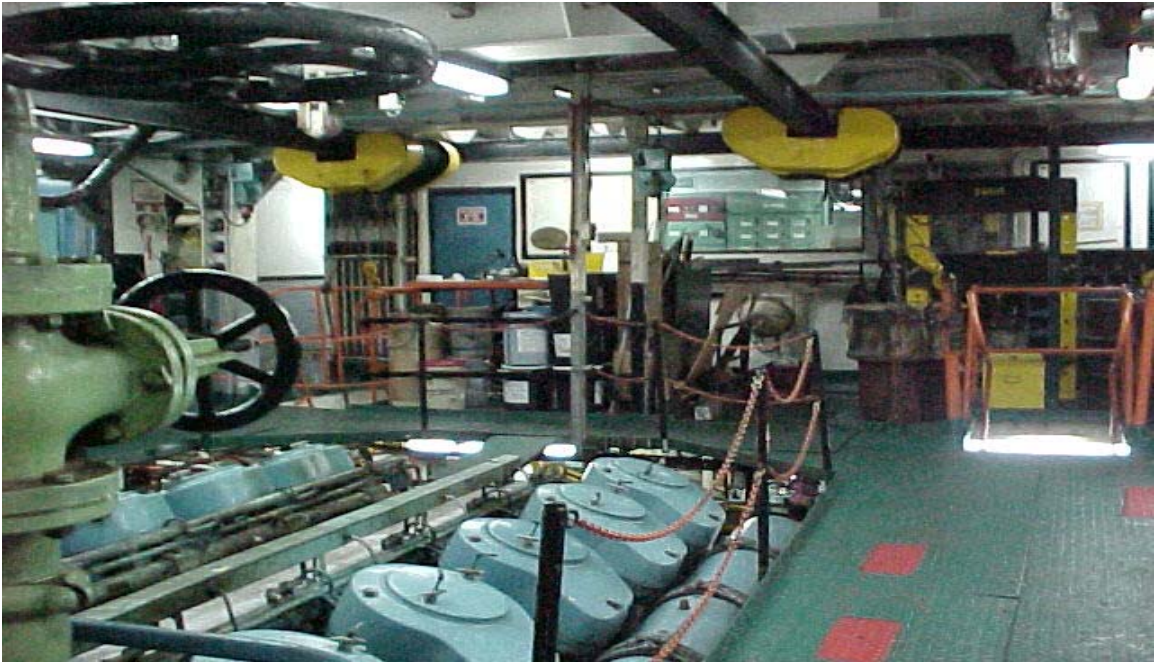
M.V. Cabot Engine Room (upper level, aft starboard)
