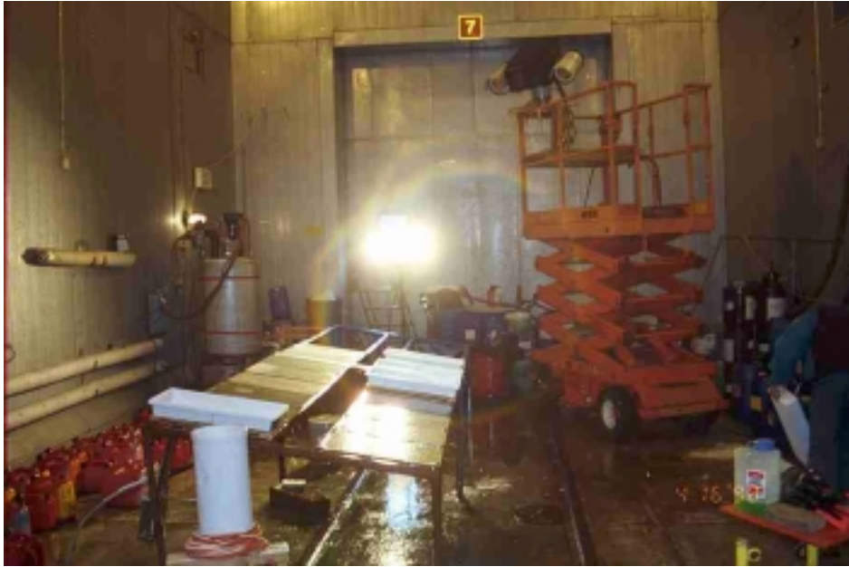
Photo 3.5: Interior View of the NRC CEF
