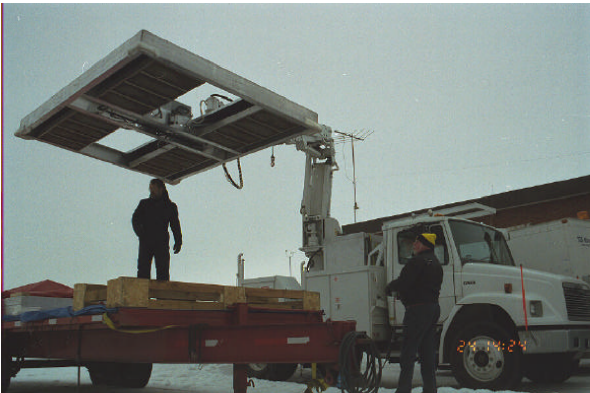
Photo 2.2 Heater Panel on Truck Boom
