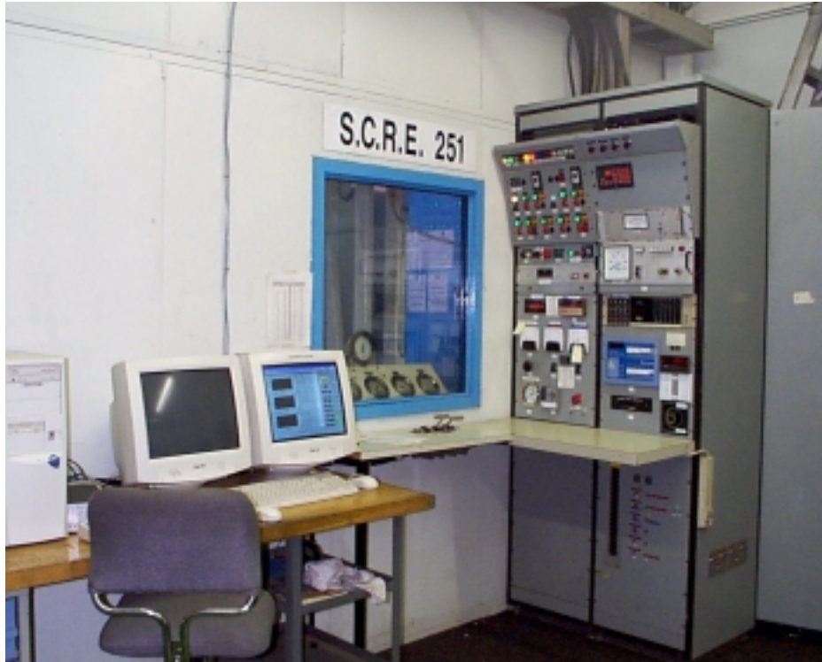
C-2: Control Unit
