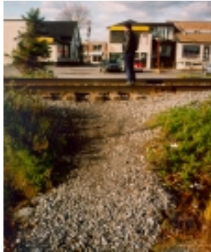
Track without ballast Rails could buckle
