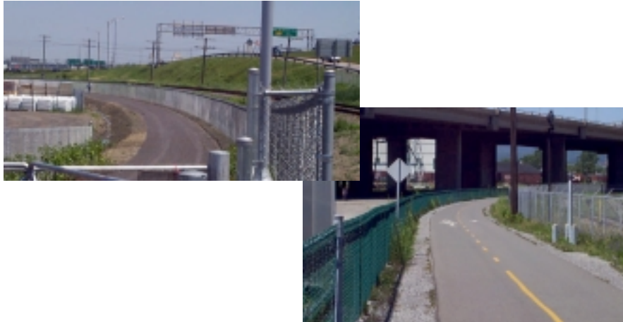
Land purchased from the railway for the construction of a bike-foot path
