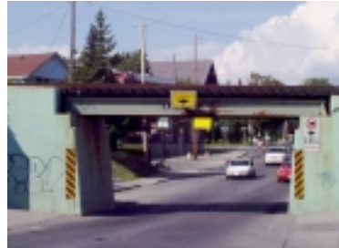
Wrong colour used to indicate clearance height
