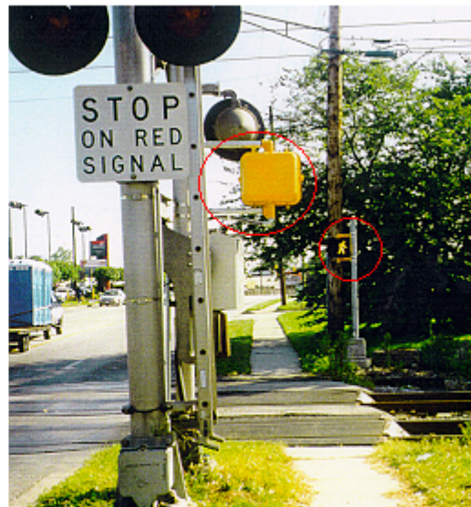
PEDESTRIAN SIGNALS - SOUTH SIDE
