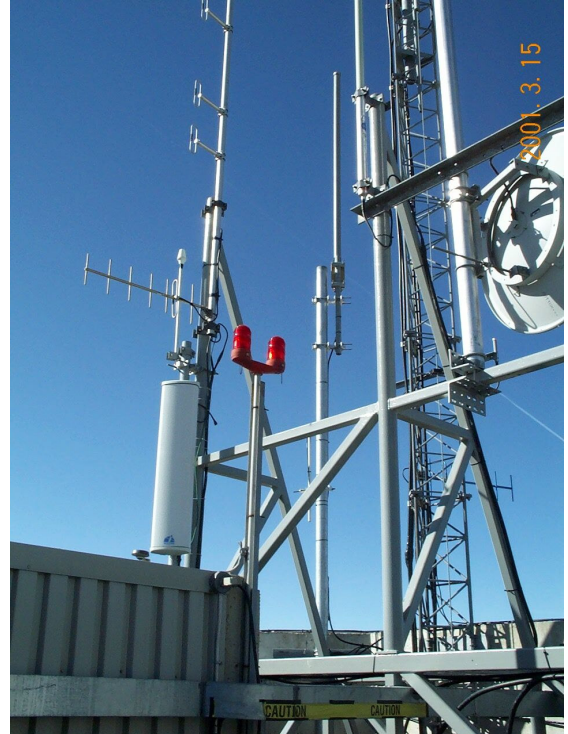
Photograph 2 - Antenna configuration on COP
