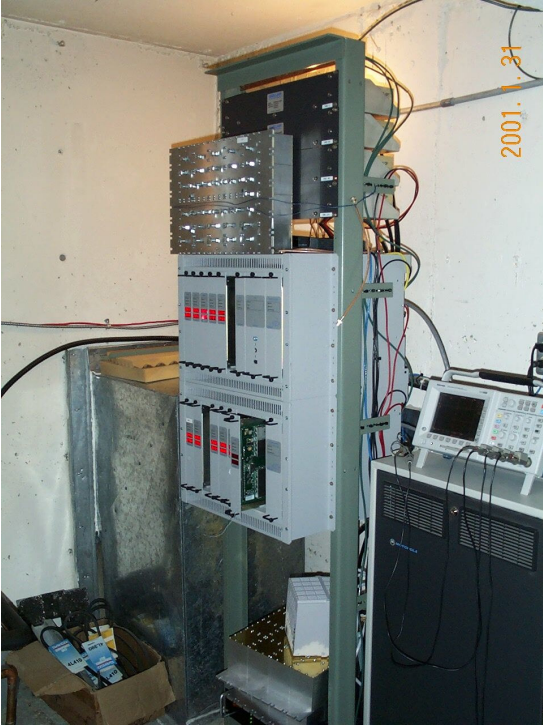
Photograph 5 - Equipment rack in Fortress site
