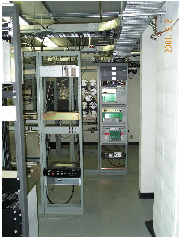
Photograph 8 - Equipment rack in tower shack
