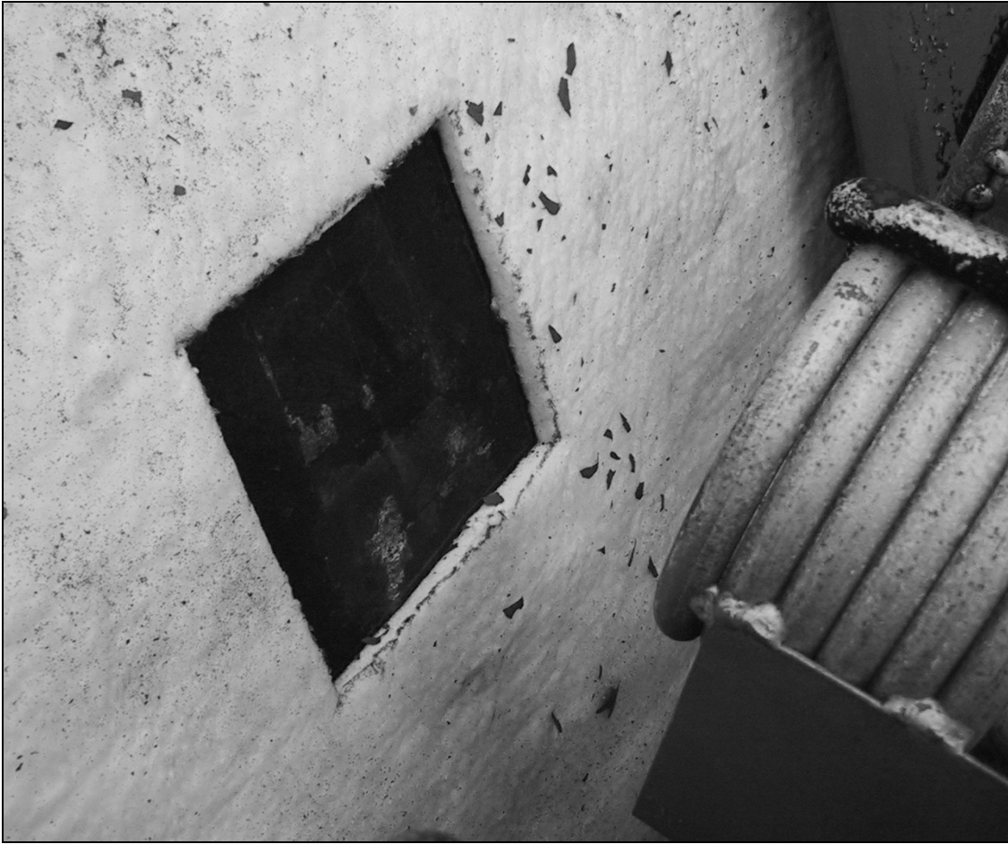
Figure 16: 15.2 cm Defect, Jacket Removed (Test 5)
