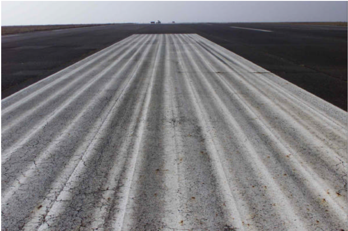
Figure 4. Overall view of touchdown paint marker
