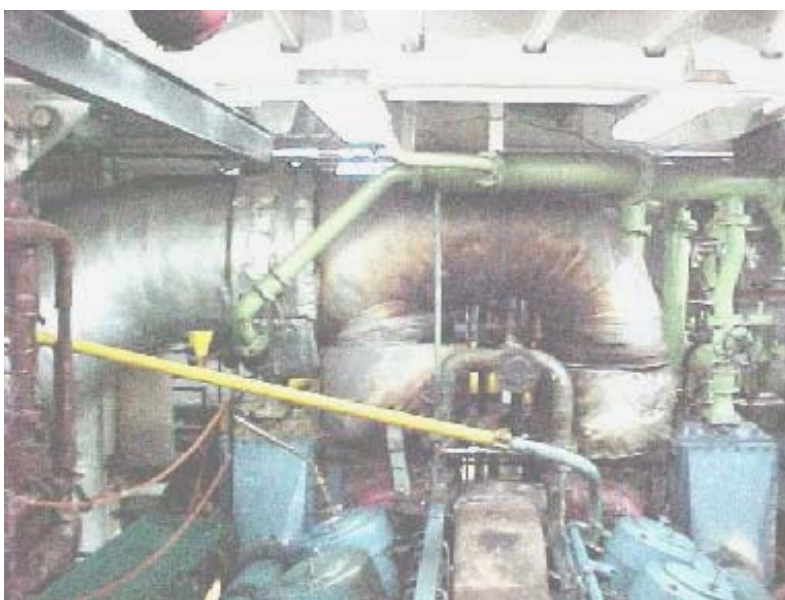
Figure 2.3 Exhaust Ducting and the Top View of the Pielstick Engine
