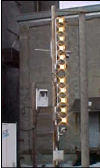
Figure 70 – Defective light bulb
