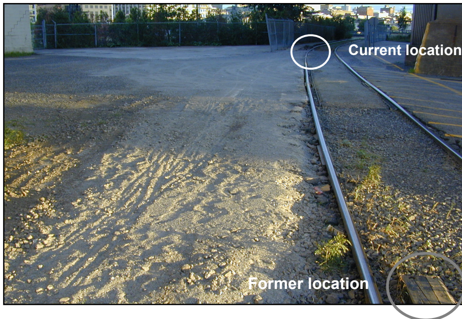
Figure 13 – Old and new location of the A/B wheel sensor
