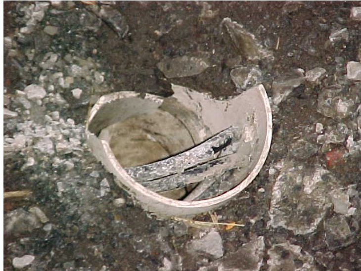
Figure 67 – Damaged Boot leg
