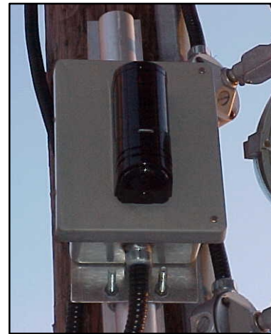
Figure 22 – Receiver on side 2
