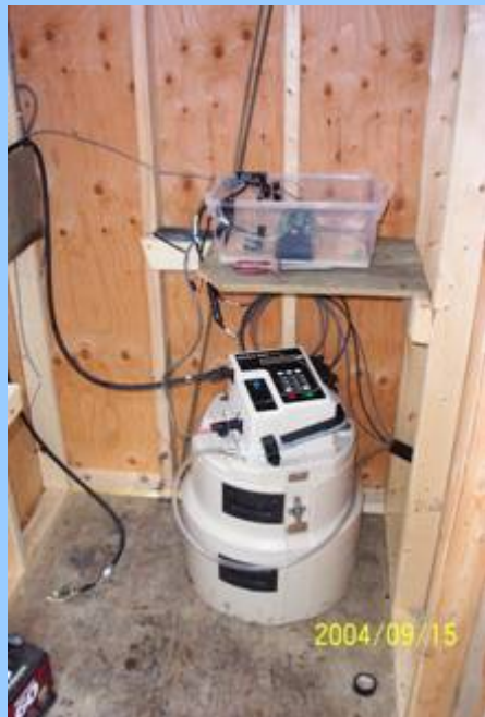
Auto-water sampler and data logger located in shed.
