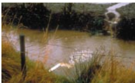
Outlet of a tile drain
