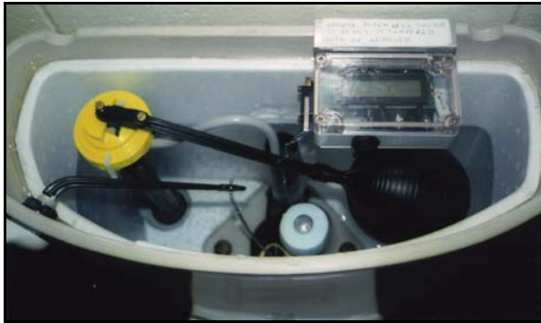
ETC Flush Counter installed under tank lid of American Standard Cadet 6 litre toilet.
