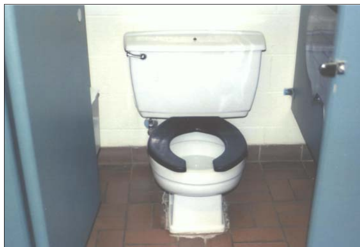
Typical 13.2 litre conventional toilet.
