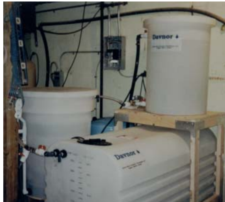
An automated slow sand filtration system, operating in demand mode, eliminates the cost of wastewater storage and handling
