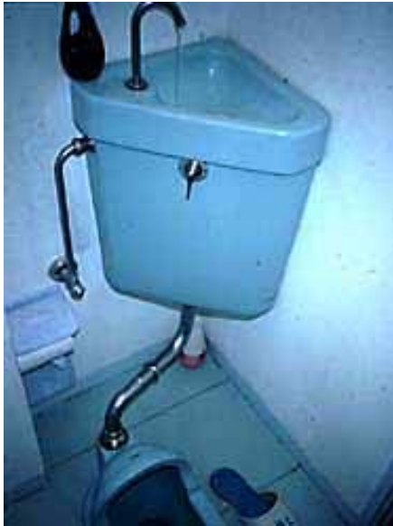
Sink (grey water) cascading to toilet
