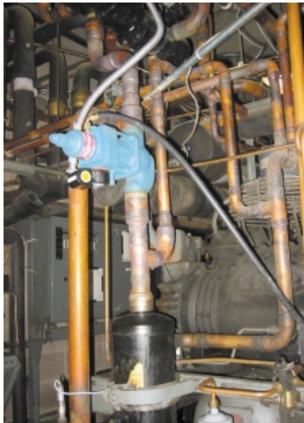
Head pressure reduction controls for refrigeration compressor system
