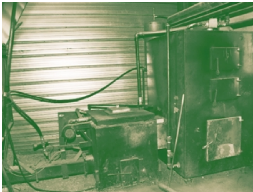
One of the two 160-kW BCSs on the Schurman Farm.
