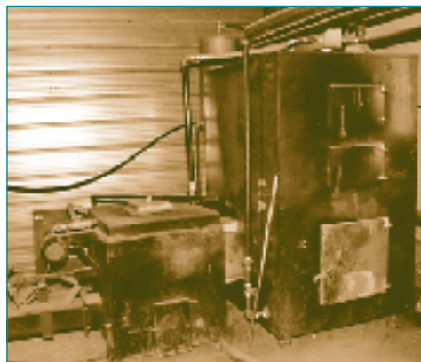
Here is one of the two 160-kW BCS on the Schurman farm.
