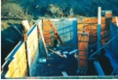
Taking the forms down at the CCHT InfoCentre after the first-ever pour of self-leveling concrete for residential basements in Canada.
