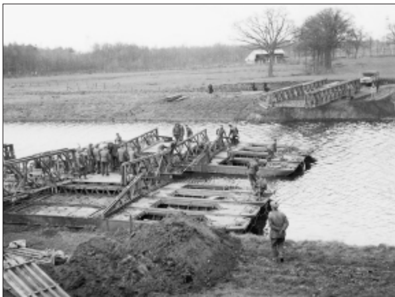
4 TH DIVISION ENGINEERS WORKING ON A BAILEY BRIDGE ACROSS THE TWENTE CANAL AT DELDEN. (NATIONAL ARCHIVES OF CANADA 49159)
