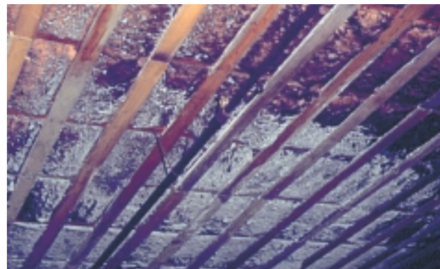
Ceiling of a cold-storage warehouse contaminated because of an accumulation of dust and condensation
