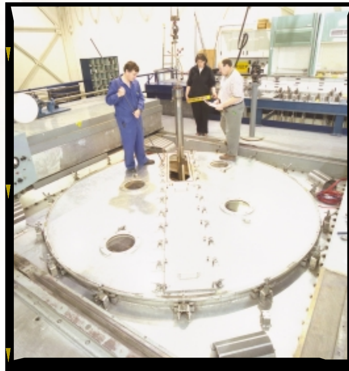
Staff from the Reactor and Radiation Physics Branch install a "hot channel" in ZED-2 allowing reactor physics measurements to take place at pressure and temperature conditions close to that of an operating CANDU power reactor. These measurements will be used for physics toolset validation.
