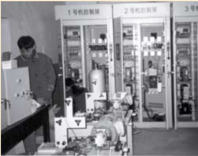
Small hydro automated control unit in China.
