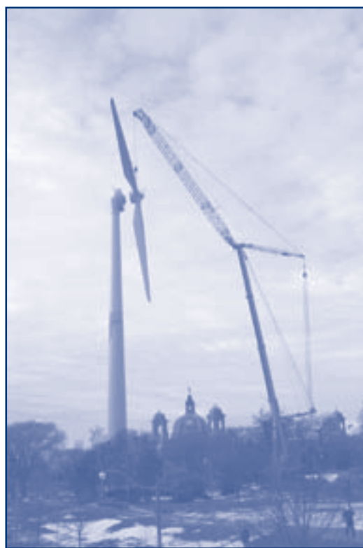
Attaching the blades to the waterfront wind-turbine at Toronto's Exhibition Place. Photo: Toronto Renewable Energy Co-operative.
